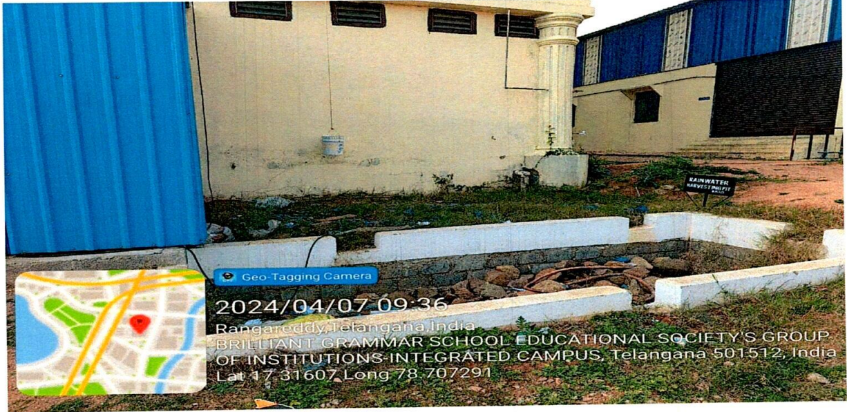
Rain water harvesting pit.
